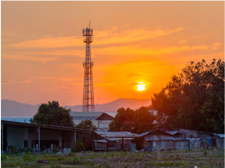
Fixed wireless internet system, with antennas that provide coverage of 30 kilometers around, very useful for rural areas or communities with infrastructure backwardness.
