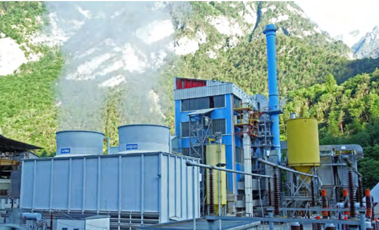
SICET biomass energy production plant in Ospitale di Cadore (Italy).
