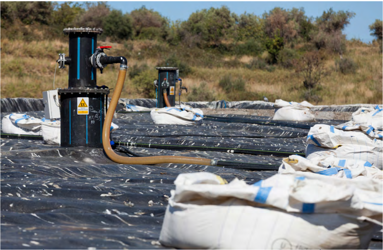
Image of a biogas plant at the Messina landfill (Italy).
